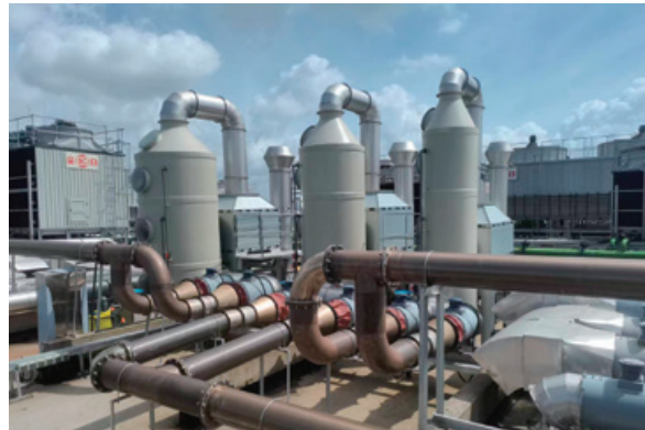
Sunny Zhejiang Optics Exhaust Gas Treatment Facilities
