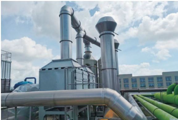
Sunny Zhejiang Optics Exhaust Gas Treatment Facilities
